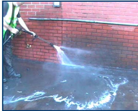
Oil had covered brick work up to 1m
